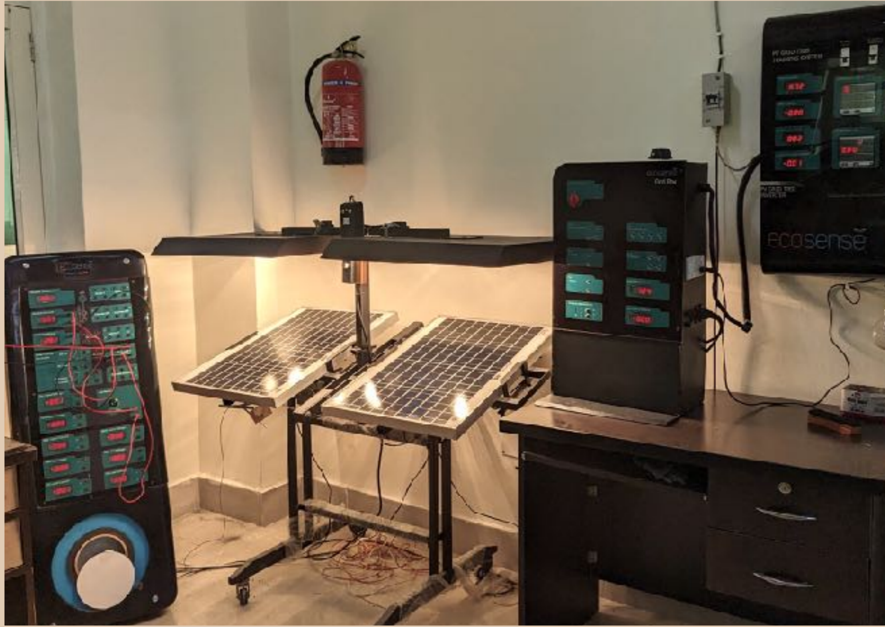
Renewable Energy Lab
