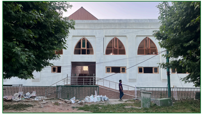
Construction of a hall with multiple washrooms for both ladies and gents
